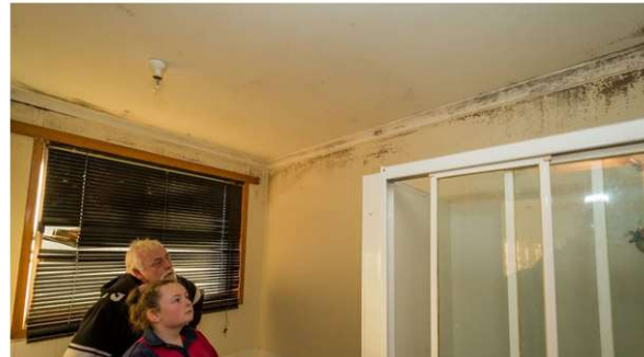
David and Taylor Kearnes inspect the interior of a Tasmania house in Trevallyn, which has been infested with mould.
