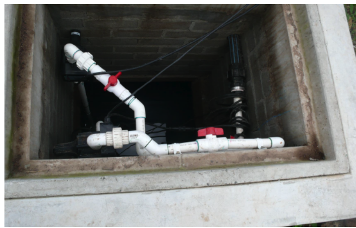
water pump and float switch
