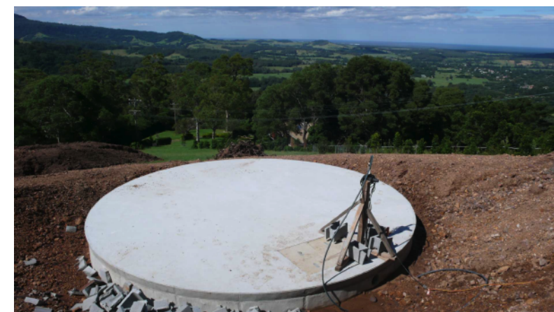
larger below ground water tank
