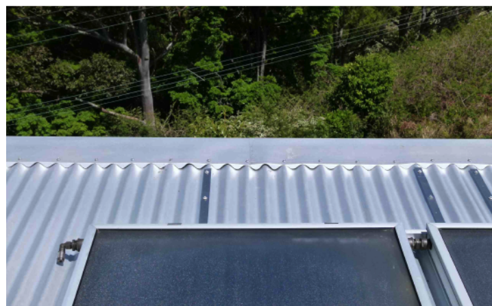
low profile roof mounted solar hot water system with gas back up
