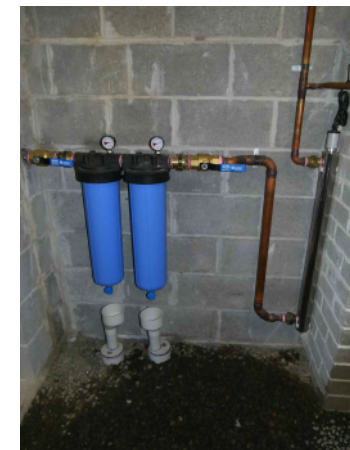
particulate filters and energy use monitoring
